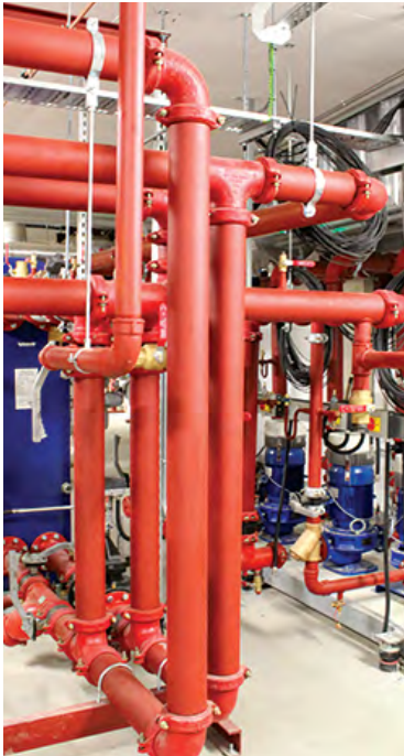
GRINNELL Mechanical Grooved HVAC System Installation
